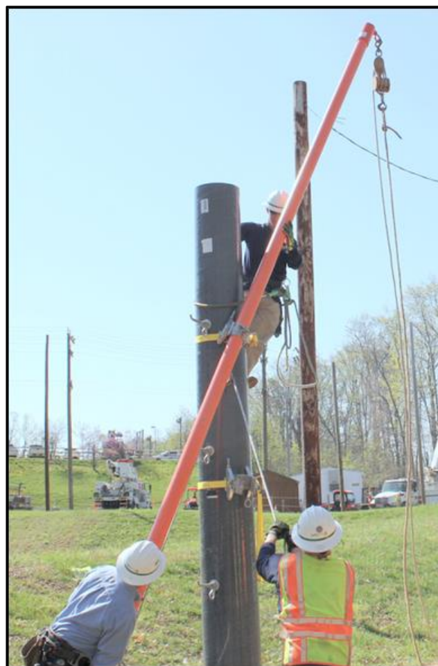
Figure 15: Sliding the gin pole through the upper clamp assembly to raise into vertical position.
