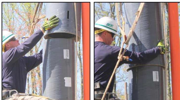
Figure 23: Keeping fingers away from pinch points, the climber gives direction to the crew while guiding the upper module onto the lower module.
