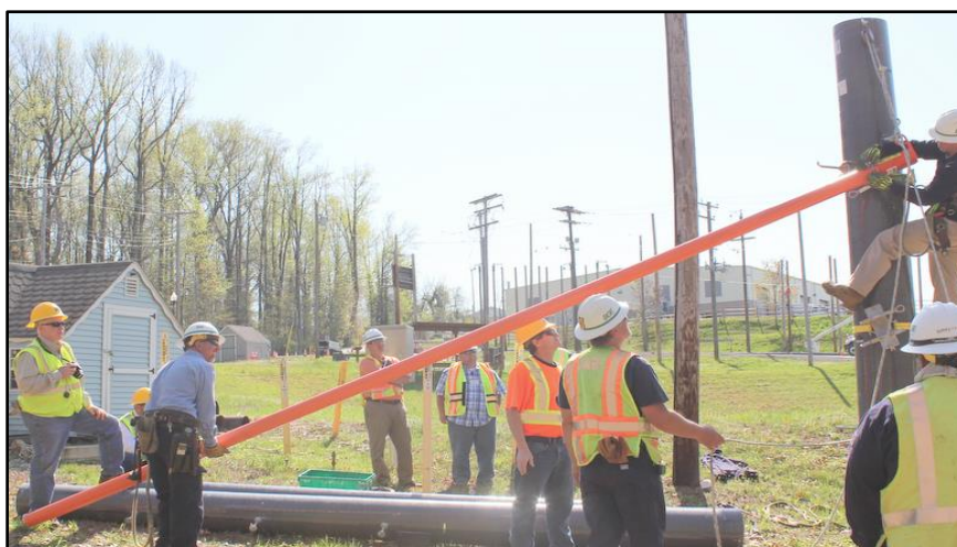
Figure 13: Climber attaches top of gin pole into the friction clamp, leaving the wing nut loose to allow the gin pole to slide into the vertical position.
