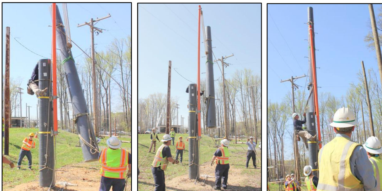
Figure 22: Crew lead is observing and directing the crew as the module is raised with a smooth consistent pull until the base has cleared the upper edge of the bottom module (far right).
