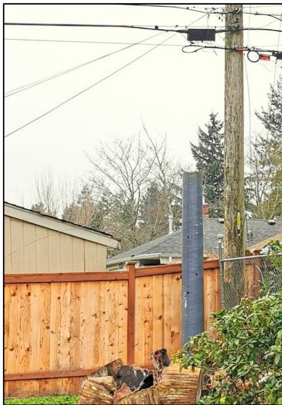
Figure 7: The base module installed in a backyard, a day prior to the planned outage.
