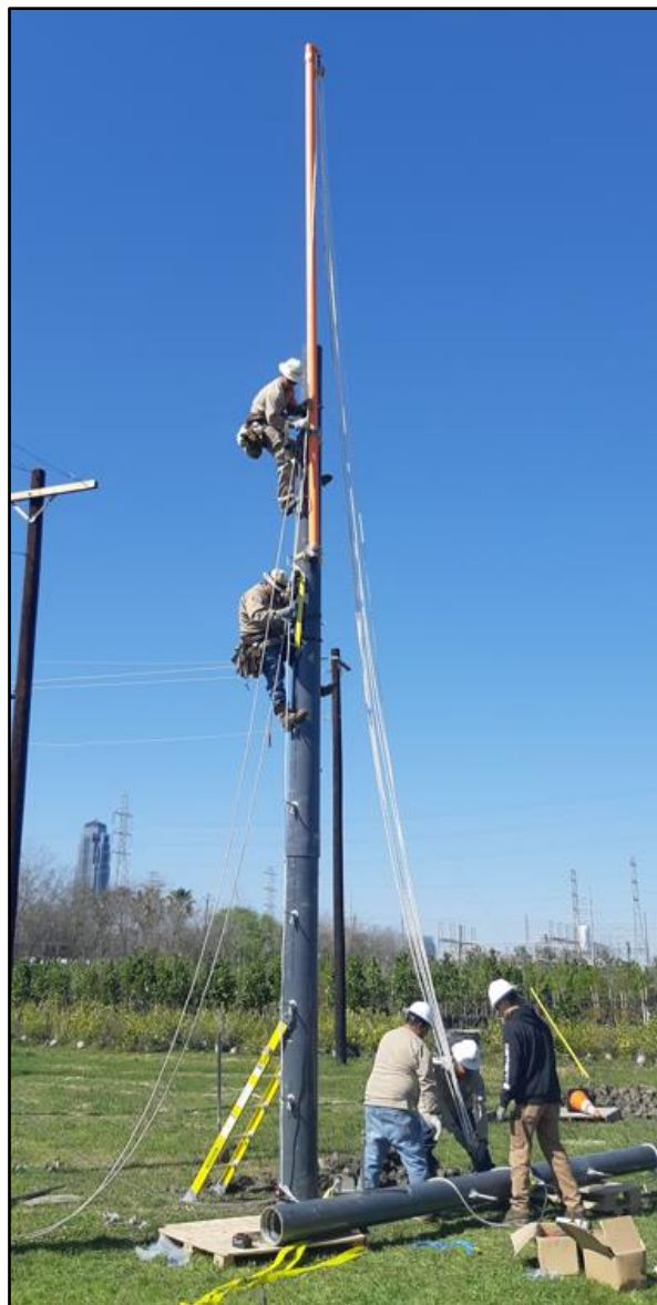
Figure 1: Line crew preparing to lift third section (RSM-02) of a 50 ft. [15.2 m] pole at a training center in Texas, USA.
