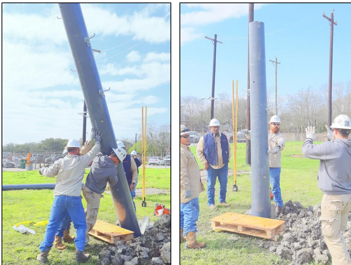
Figure 8: Setting the base module with steps pre-installed (left). Rotating the base for proper alignment (right).
