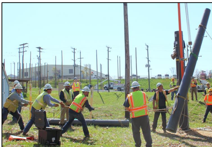
Figure 21: Three workers pull hand over hand, raising the module, while listening for directions from the observer.
