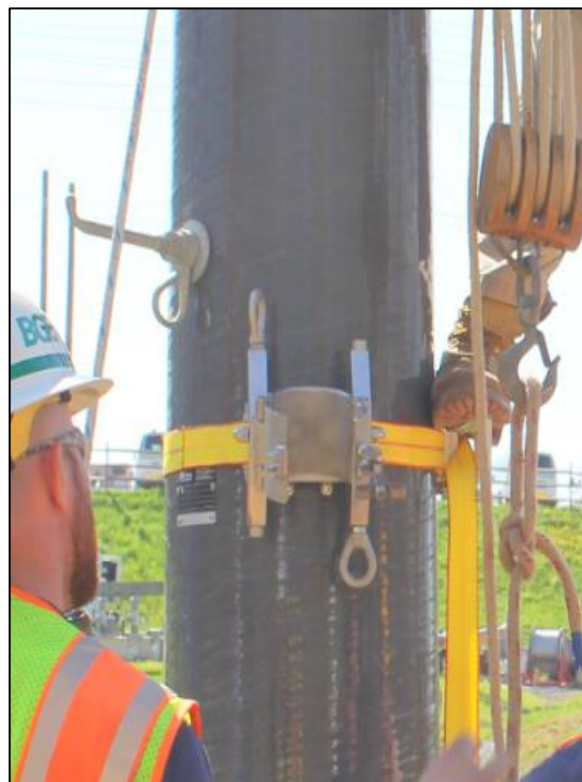
Figure 3: Climbing Steps on the B and D Axis. Clamp Assembly on the E Axis, which becomes the Gin Axis for this Installation.
