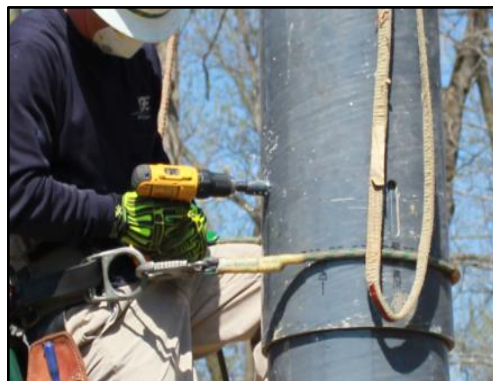
Figure 26: Chase drilling the hole for a climbing step after the joint is compressed.
