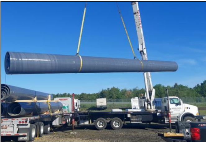
Figure 8: Transporting a 90 ft. [27m] nested pole set to its off-road installation location.
