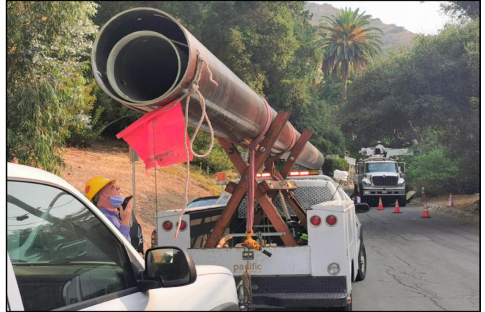
Figure 16: A 50 ft. [15m] nested pole set secured on a 1-ton truck easily navigates up a windy road in Burbank CA.
