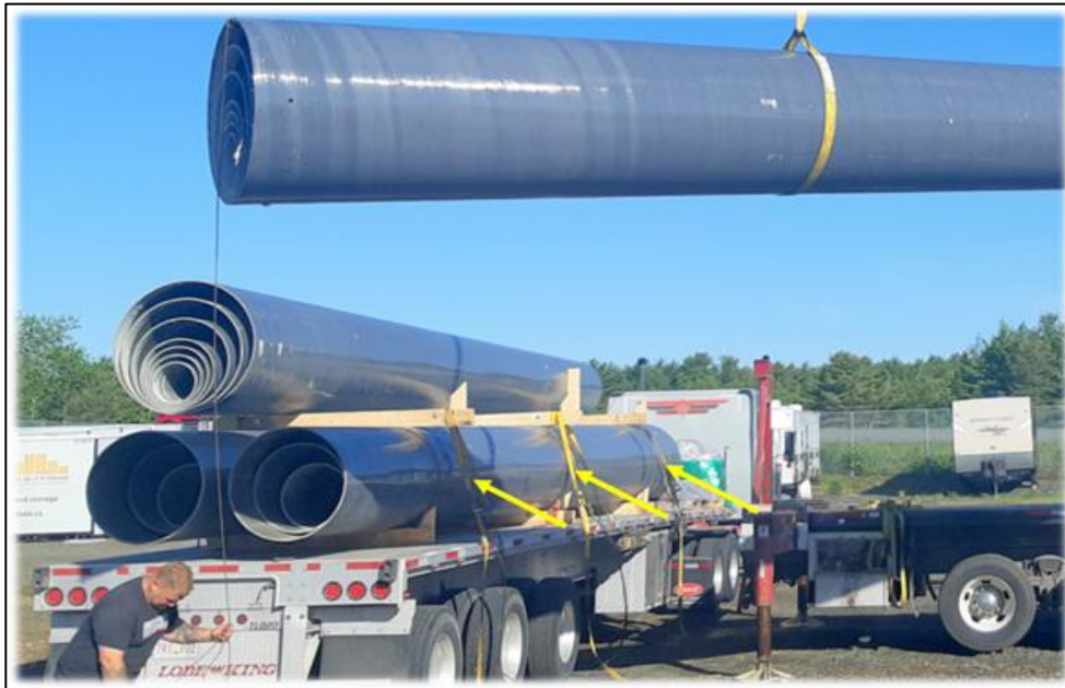
Figure 7: Added cargo straps secure adjacent pole set prior to unloading first pole set.
