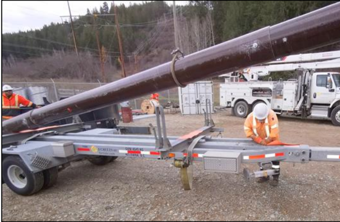
Figure 15: Strips of an old rubber blanket lay between the steel trailer bed and smooth RS Pole.
