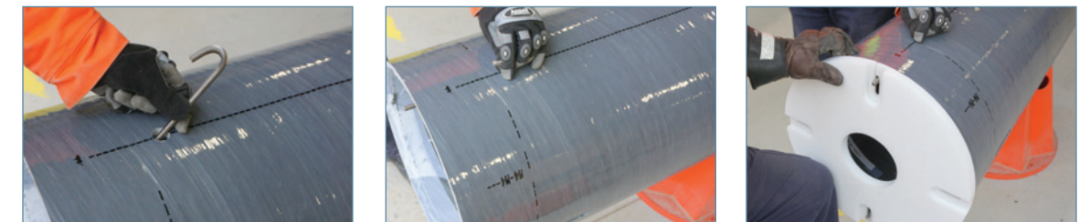
Figure 19a, 19b and 19c: Installing a J-Bolt into the Pre-Drilled Hole and Positioning the Base Plate
