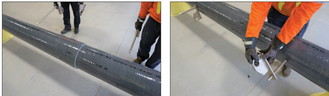
Figures 9a and 9b: Inserting the Jacking Bars and Adding the Jacking Plate
