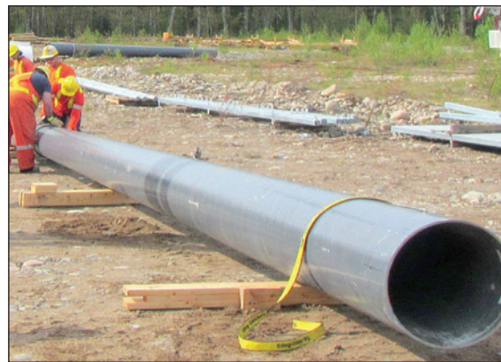
Figure 5a: An RS Pole on Wood Dunnage
