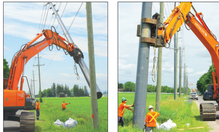
Figures 25a and 25b: A Pole Setter Setting a Double Circuit 44kV Pole During an Outage
