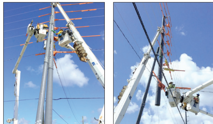
Figures 30a and 30b: Base Module Being Replaced Using Live Line Techniques
