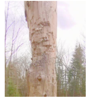
Figure 6: Wood pole damaged by a bear.
