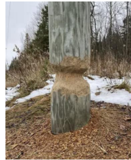
Figure 5: Wood pole damaged by a beaver.
